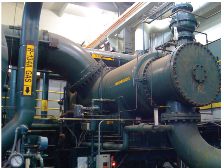
Figure 8.18: Chiller in the University of Notre Dame power plant, 14 June 2010.
